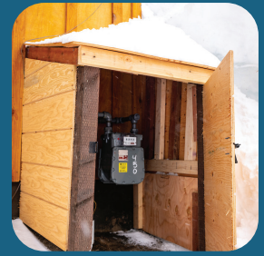
METER WITH SNOW SHELTER
